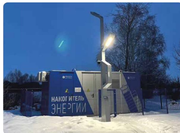
Energy Storage System
