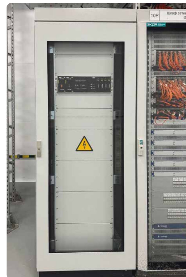
External view of the panel installed at the Sputnik 110 kV substation.
